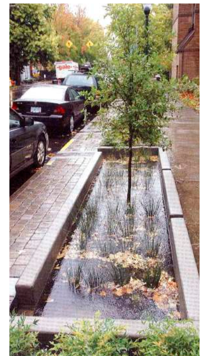
Water harvesting along streets
